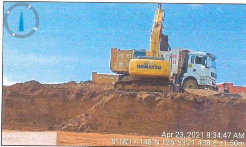
Figure 6-4. Backhoe loading the ore into the 18-tonne capacity dump truck to be transported to the stockpile area.
